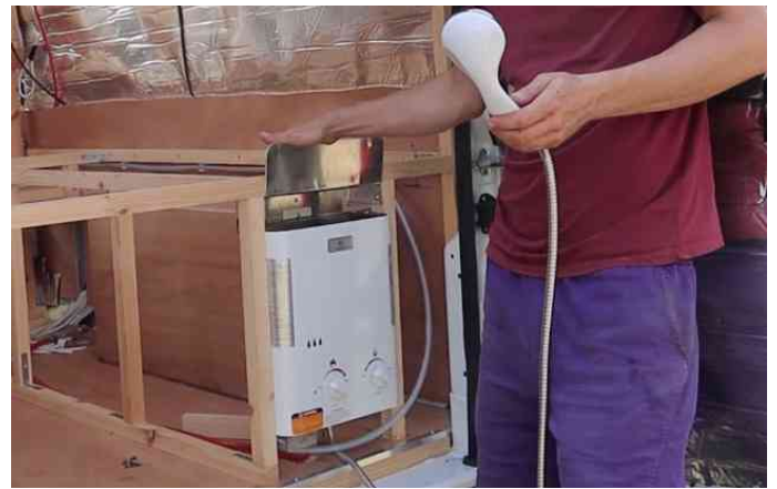
The gas-powered shower being installed (it can only be used when the back doors are open).
